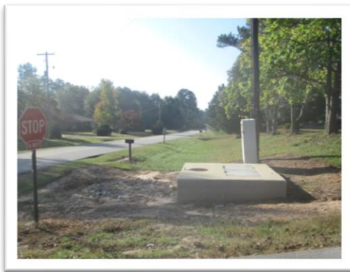
Booster Pump Station at Montville Road and Boyd Road
