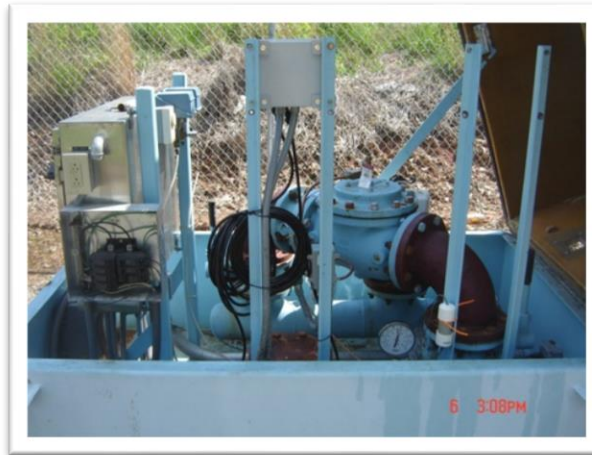
Pump Station Converted to Pressure Control Valve
