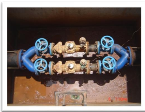
Meters at LaGrange Connection
