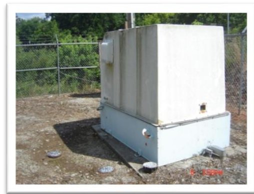
Pump Station Converted to Pressure Control Valve
